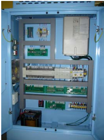
PLC MITSUBISHI FX2N CONTROLLER - SIMPLEX
