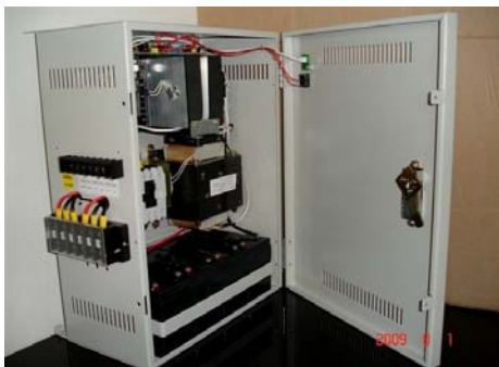
UPS "UNI POWER" TAIWAN AUTOMATIC RESCUE DEVICE
