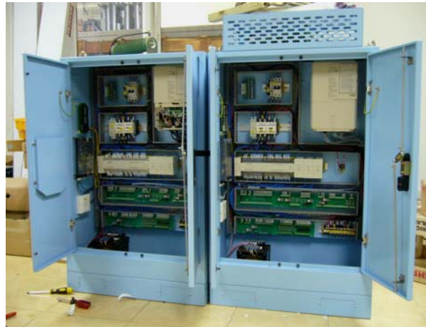
PLC MITSUBISHI FX2N CONTROLLER - DUPLEX (2 CAR GROUP)
